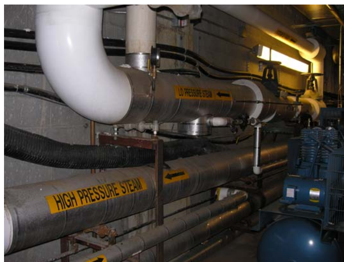
Utility lines through the Basement
