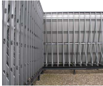
(Left) Roof Screen Wall Framing Detail (Above) Roof Screen Wall and roofing system
